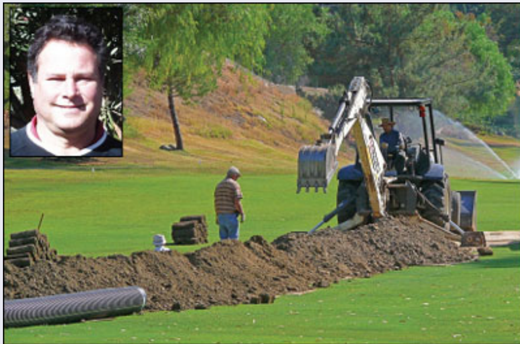
A drainage project to eliminate drainage issues on holes #4, #5, #6 and #7 will take a few more weeks to complete but will greatly improve the course. Here, drain pipes are installed in the fifth fairway.
